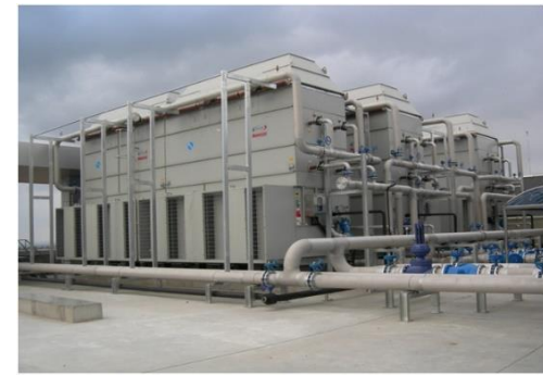
“P사” 전산센터 Cooling Tower
