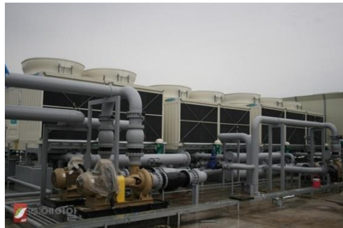
“H사” 전산센터 Cooling Tower
