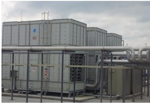
“P사” IDC Cooling Tower
