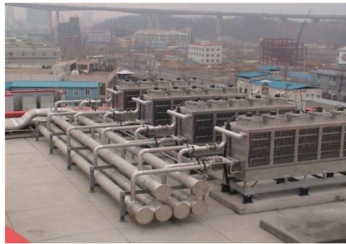
“K사” 전산센터 Cooling Tower
